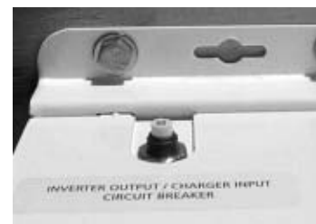
Circuit Breaker Reset
