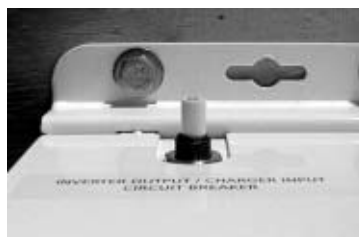
Circuit Breaker Open
