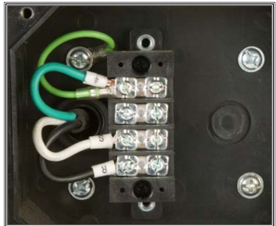
Figure 106. Power connection junction box.
