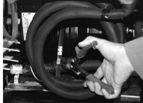
Cutting band that is around compressor
