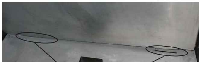
Slots on floor of firebox base.
