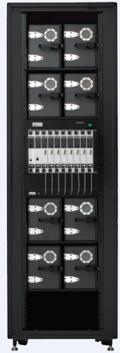
8 STE2900's installed in a Veriwave dense-pack test rack
