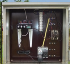
AR2 & AR2L Mounted in an outdoor enclosure with 110V lighting relay controls
