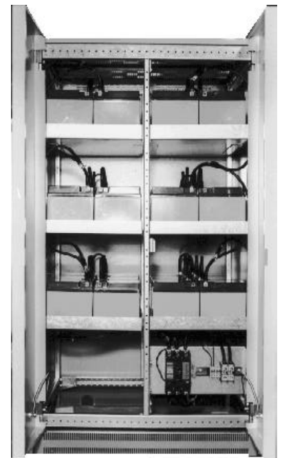
FIG. 1.12.4 Battery cabinet B3/38
