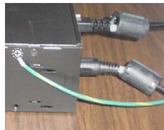
This partial view of the data acquisition device shows its connection to the ground-line. It also shows two ferrite collars, the foremost of which is clamped to the power cable. The background collar is clamped onto the Ethernet cable.
