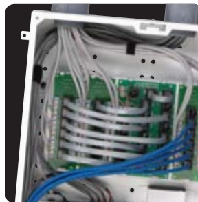
HOME WIRING & NETWORKING
