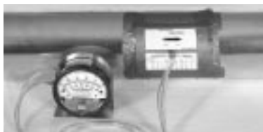
figure 11.5 Avoid leakage by sealing air flow grid in duct with duct tape.
