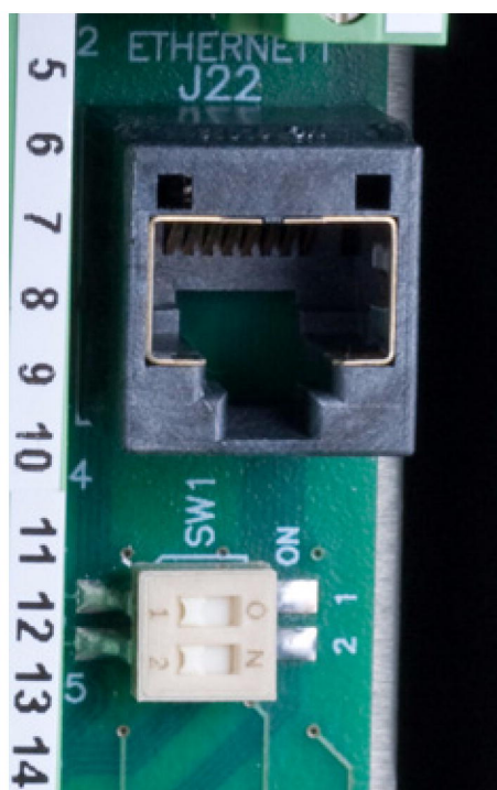
Figure 3-11: SW1 switches on the back plane
