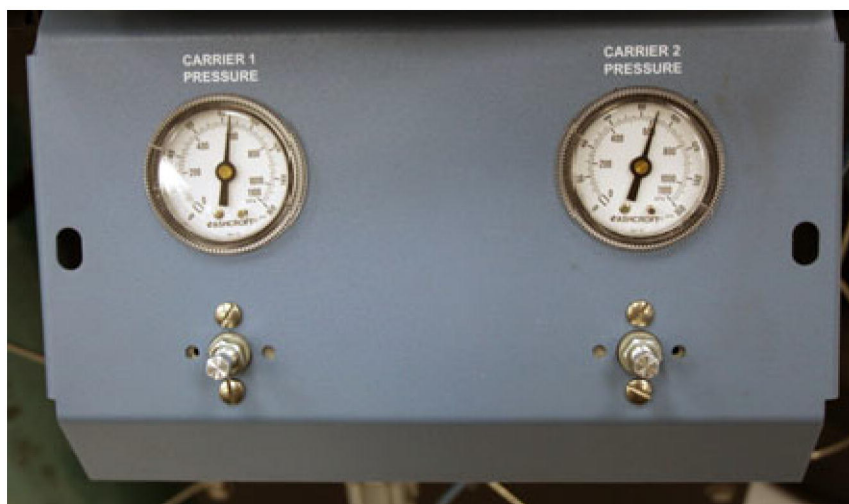
Figure 2-8: The mechanical pressure regulators
