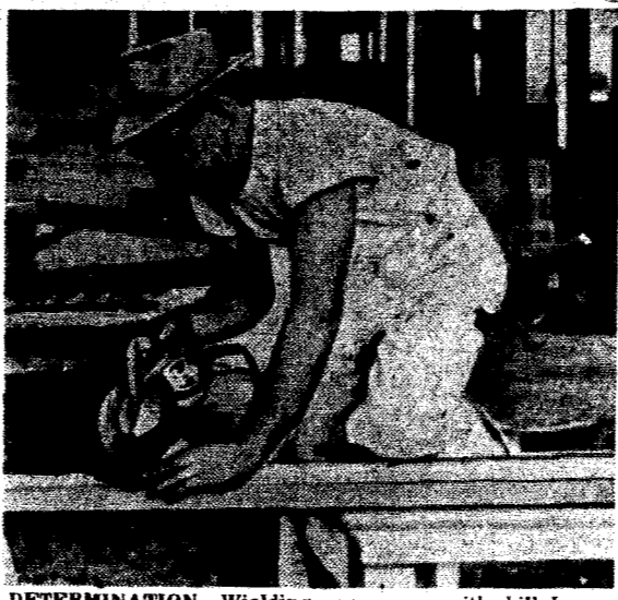
DETERMINATION —Welding a power saw with skill, Leonard Stuh, 43, of Turner, Ore., is building his own house. The blind ex-GI does all the work himself, using several power tools, with occasional help from his son Billy, 15. Prior to his blindness, he had never handled power tools.
