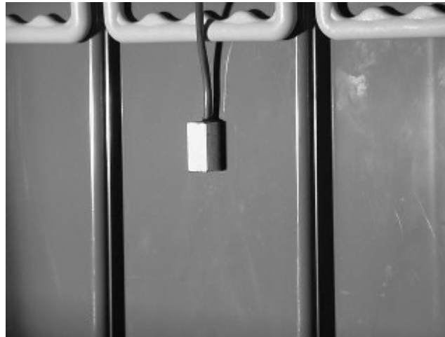
Figure 3.8-3 Typical location of Battery Temperature Probe
